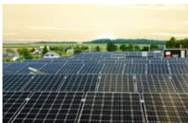
Installation photovoltaïque de 30 kWc
